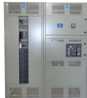
circuit breaker switchboard
