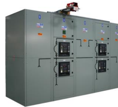
draw out circuit breakers with mimic bus and lifter
